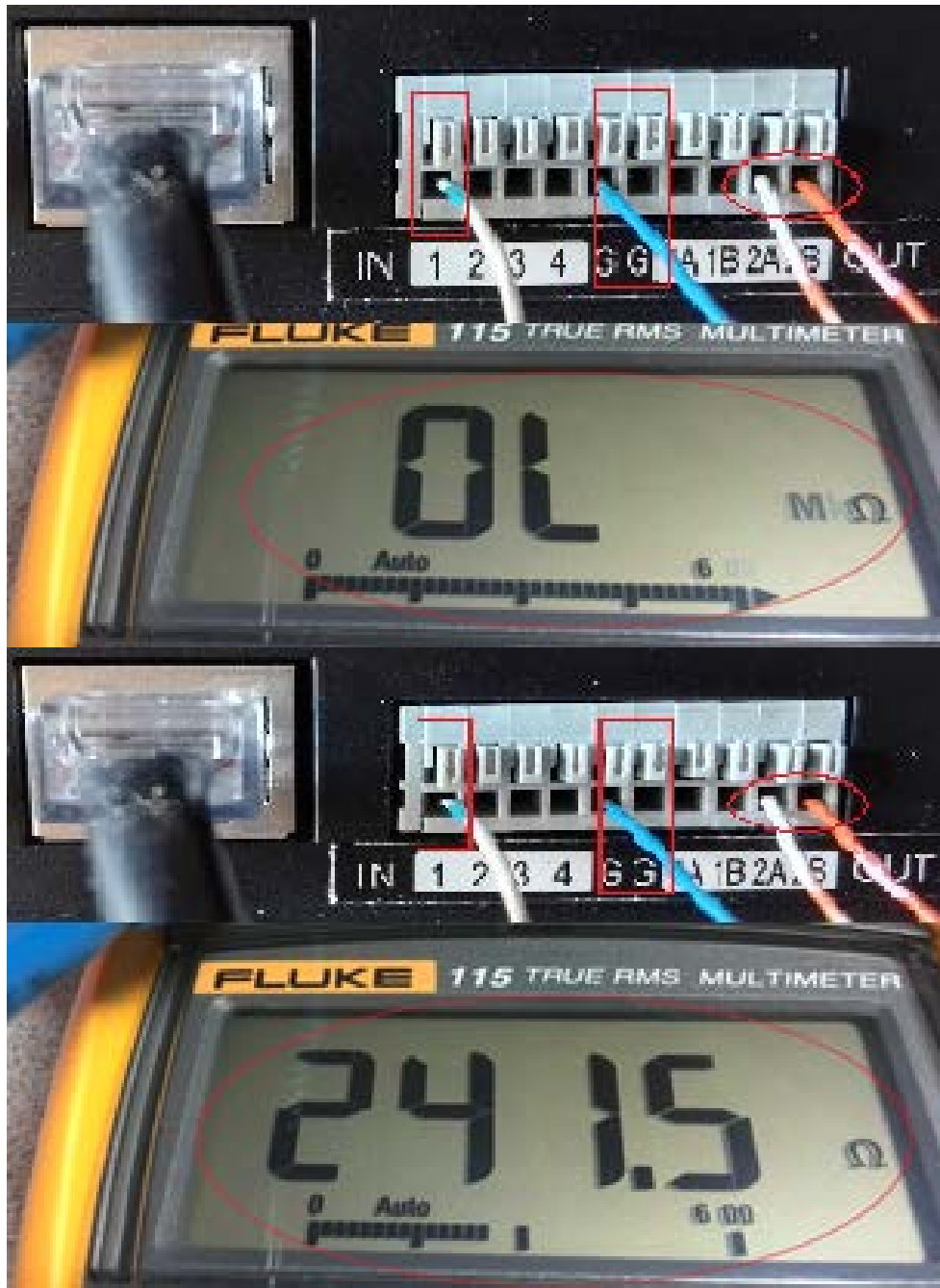
Figure 25-4: GVR355X Alarm_Out Circuit Measurement
